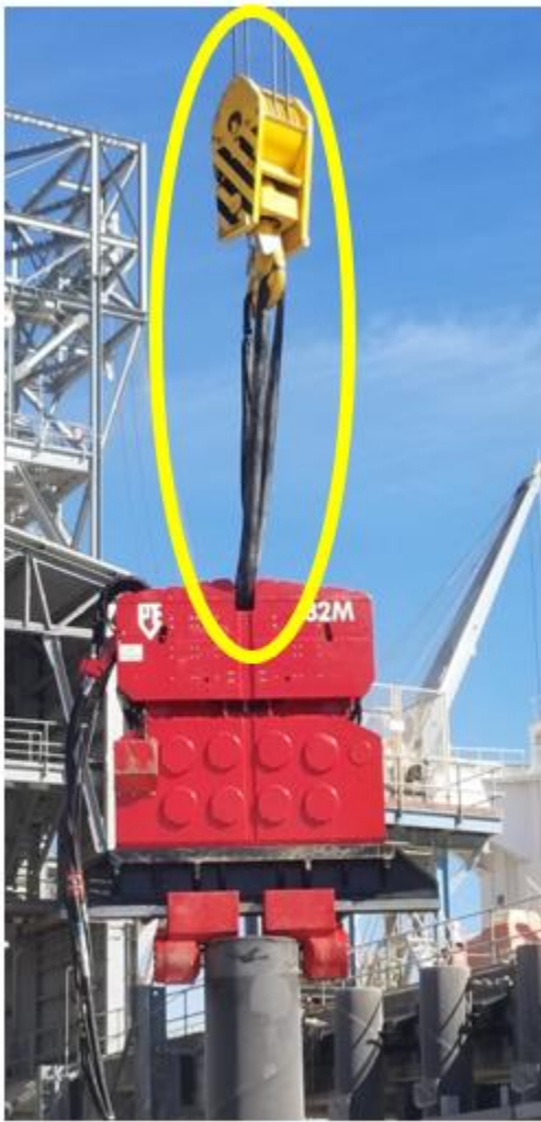
Improper: Nylon Rigging
