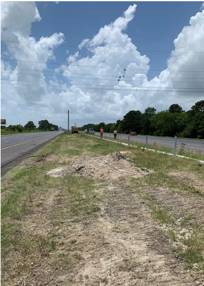
A view of the power lines from where the casing pipe was staged.
