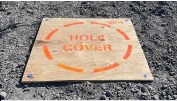
Example 1: Labeled Hole Cover 48"x48" 3/4" plywood secured with 12" anchor spikes and washers.
