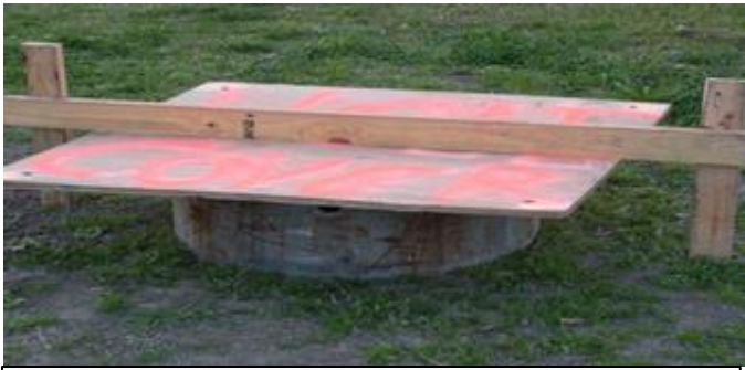
Example 2: Labeled Hole Cover 48"x48" 3/4" plywood with 2x4 secured across the top and held in place by two 2x4 stakes.
